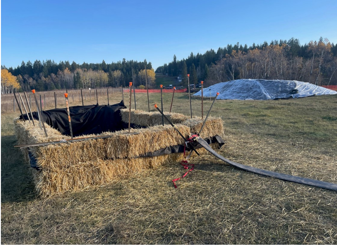
Topsoil preservation and erosion and sediment control at an outlet point.
